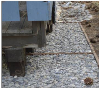
Gravel area under a gutterless roof
